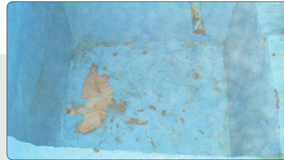
Cracked surface for Concrete water tank after 3 years installation
