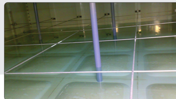
Inside state of SNB GRP Water tank after 3 years installation
