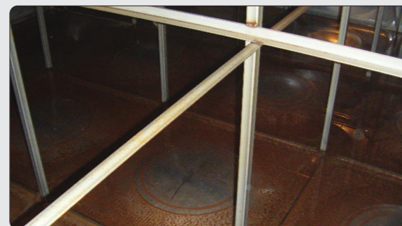
Rusted steel for STS Water tank after 3 years installation
