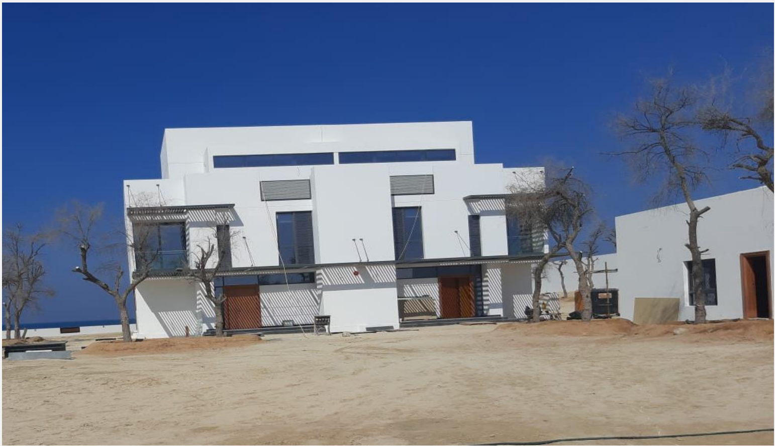
Project: PROPOSED G + 1 + R + SB 2Villas, Hamriya West, Sharjah. Owner: Stars Development Co. Job: MEP Works
